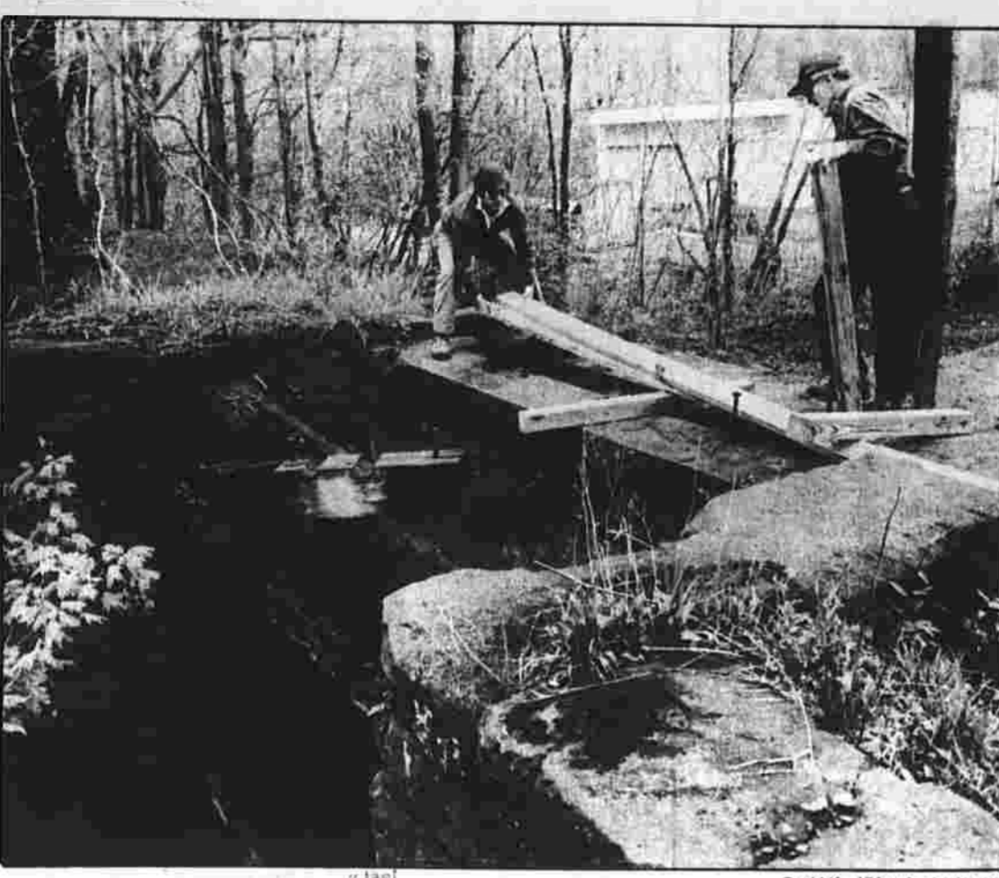
NEW BRIDGE — Steve Deureaux of Manchester, left, and John Hartoon of East Hartford get lumber ready for a bridge that volunteers built Saturday on one of the trails in the Hockanum River Linear Park trail system. The bridge goes over an old waterway behind the Adams Mill Restaurant on Adams Street. Before the bridge was built, the only way to cross the waterway was to walk on a narrow concrete wall.
